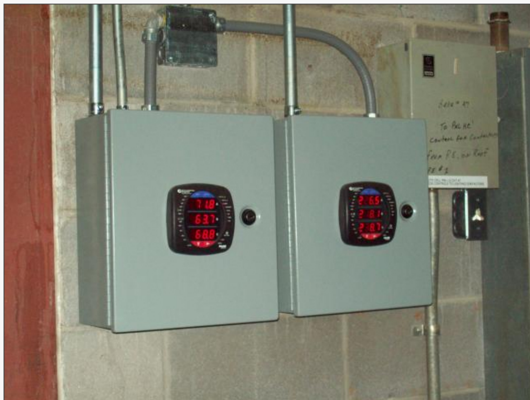
Shark 200 Advanced Electric Meters are used to capture the electric usage. In addition to electric usage data the meters also collect natural gas consumption for reporting to the Directorate of Public Works energy manager.
