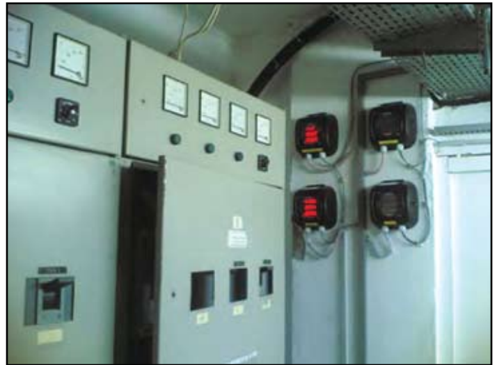
Shark®100-S submeters installed in the hospital
